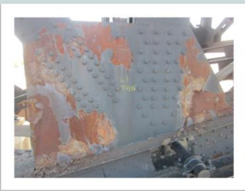
Figure 5 Deteriorated Horizontal Connection Plate
