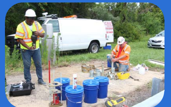
AID Material Testing Team Performing QA Testing for FDR on Rt. 55 SB (on the left: Ahmed Mohamed, Engineer, measuring moisture content using Speedy Moisture Tester AASHTO T-217; on the Right: Dan Nero, Senior Technician, molding FDR Samples for compressive strength)
