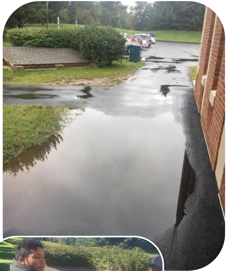
Drainage problem (Source: ASHE Scanner)
