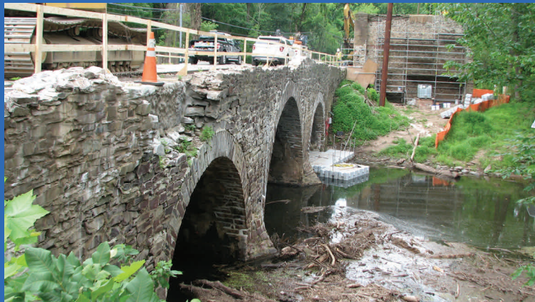
Partial collapse of the stone parapet and spandrel wall of the Stone Arch Bridge. Worth's Mill Ruin Wall is on the right.
