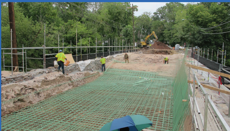
Construction of concrete saddles to strengthen the arches of the Stone Arch Bridge.
