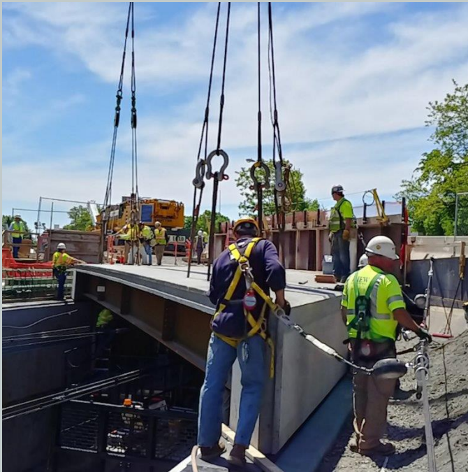
Prefabricated superstructure units were utilized to improve quality, increase safety, minimize disruption of NJ TRANSIT operations,
