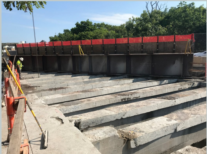
Use of a strong-back girder facilitated staged construction by maintaining the structural system's integrity, and allowed continued use of the bridge by vehicular and pedestrian traffic.
