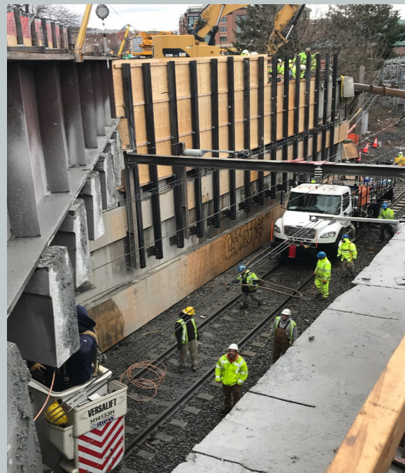
The rehabilitation successfully minimized impacts to railroad operations by continuously coordinating with NJ TRANSIT.
